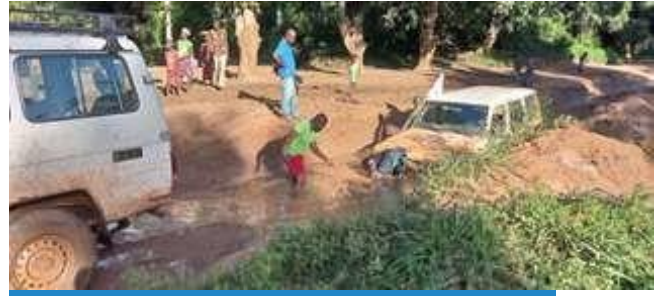
Deteriorated state of the Dimbi-Alindao road, July 2023.
